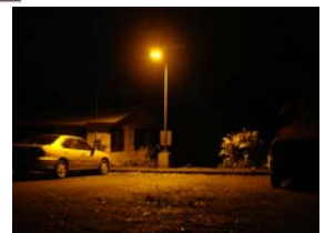
PVATUS Off-Grid Solar Powered LPS Lighting Systems Installed at the Hawaii Department of Education Honokaa Teacher Cottage on the Big Island
